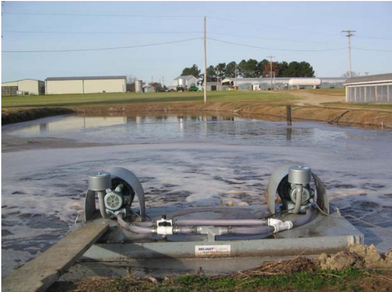
Figure 2: Reliant Model WQA Water Moving Aerator located in one end of the hog lagoon. Photo was taken approximately 15 days after aerator startup.
